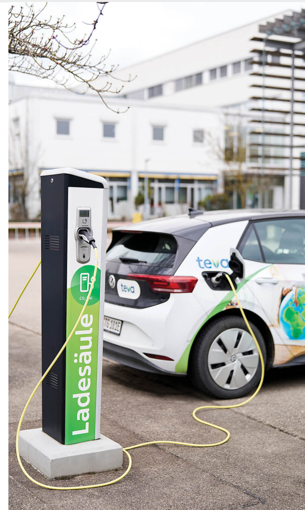
Teva electric car charging point in Germany
